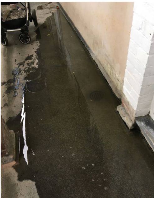
Flooding in the external galleries of the maisonette blocks.
