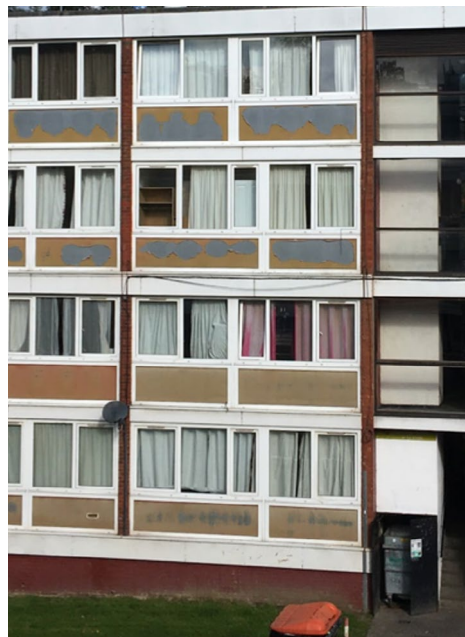
Façade showing the panels below the windows, the slabs and parts of the façades that need to be repainted.
